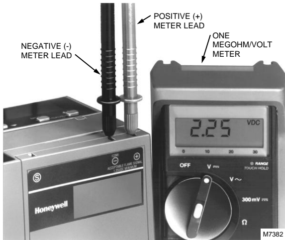
Fig. 12. Measuring flame signal voltage of 7800 SERIES controls.
